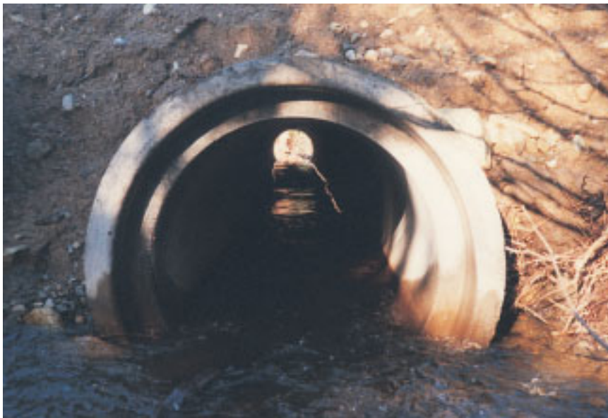
A bad design of culvert that would prevent the passage of fish.
